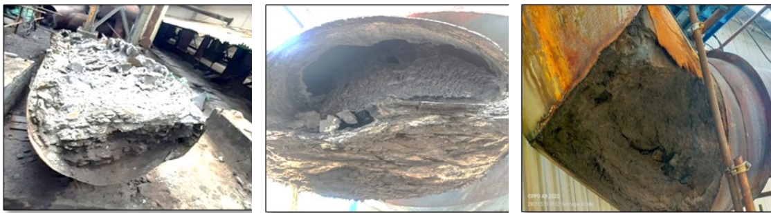
Figure 1. Jammed fume ducts.
